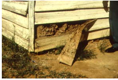
(a) Termite damage to external cladding
