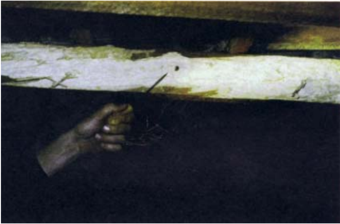
(c) Damage caused by Hylotrupes bajulus
