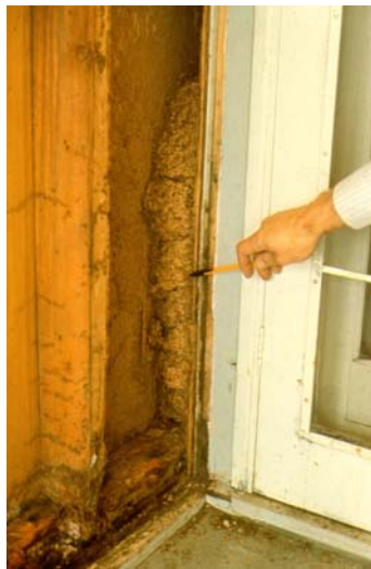
(b) Door jamb damaged by Coptotermes frenchi
